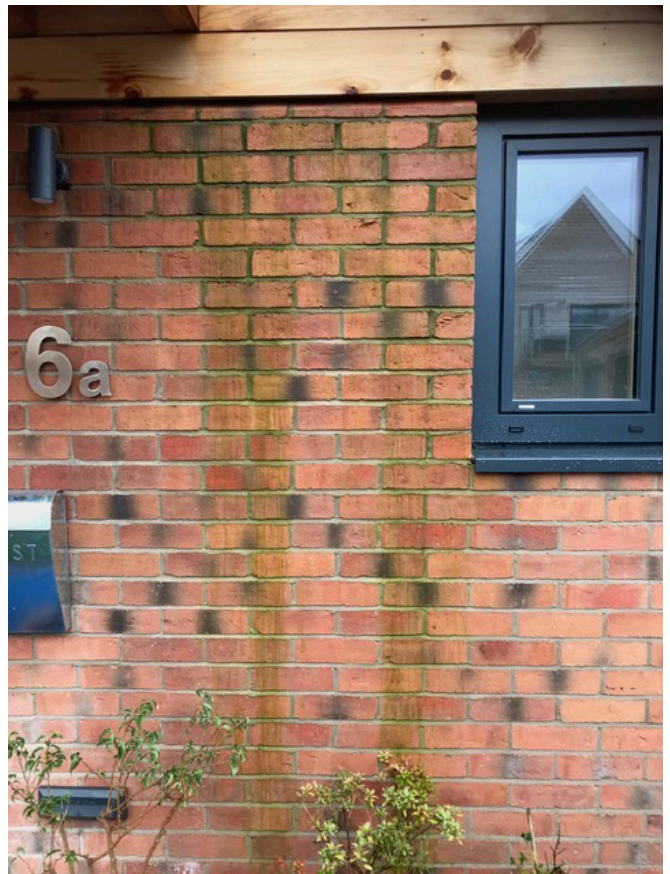
Vegetation staining due to lack of drip detail from timber cladding
