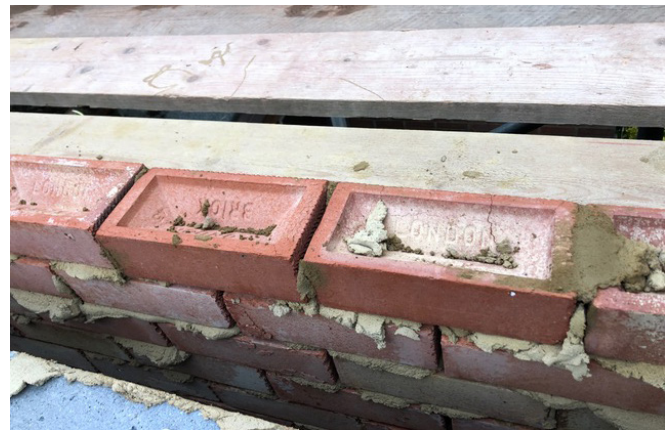
Insufficient mortar in cross joints
